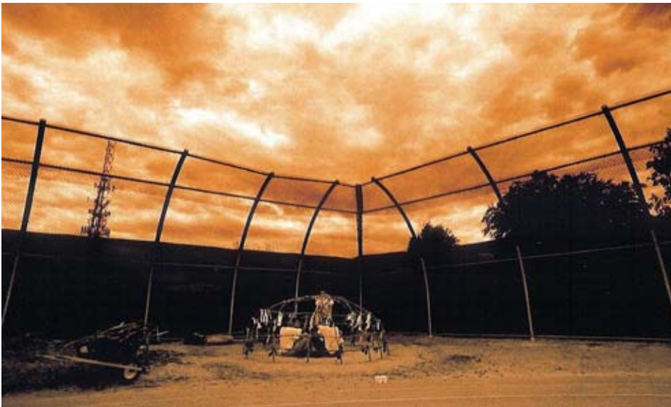
A partially constructed sweat lodge, inside the fence of a New Mexico detention center. Photo by David Michael Kennedy.
